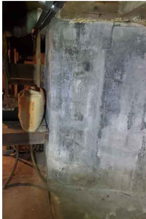
Area of foundation where poured concrete was implemented to replace original stacked stone.
