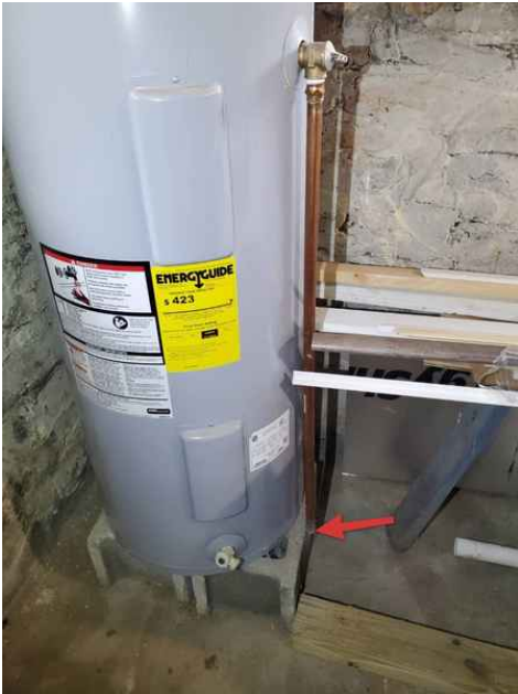
TPR Valve discharge pipe terminates 8 inches above the floor.
